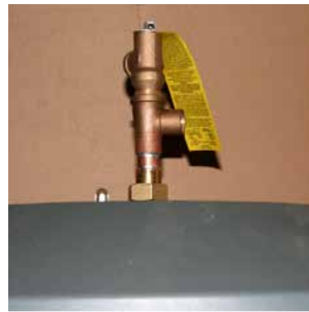
Complete assembly on SBB tank.
